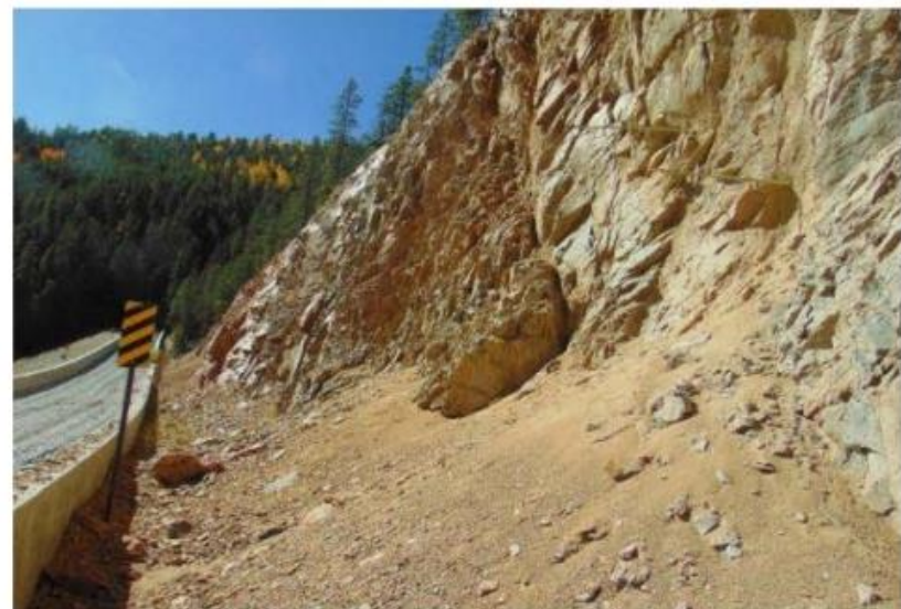
Failed rock bolts at right side photo, view to west-southwest
