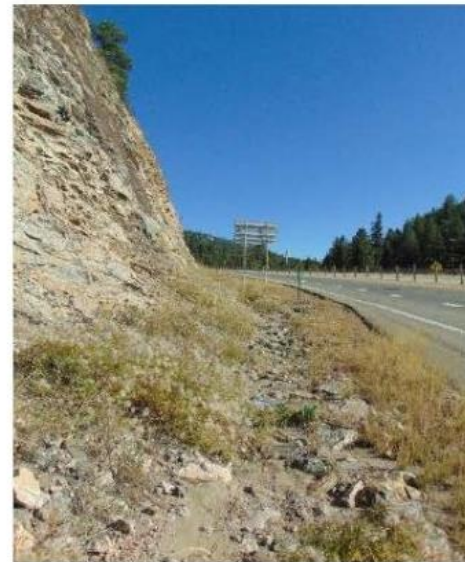
Rocks at base of cut slope
