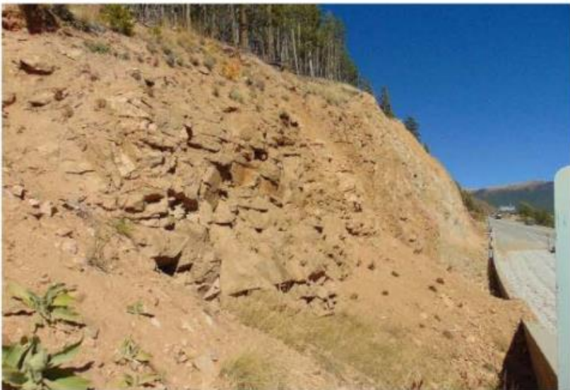
Fractured rock and loose rock on slope and behind barrier, view to east-northeast
