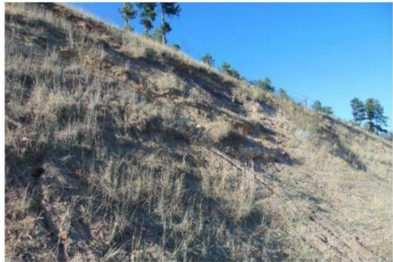
Rilling and gullying on upper soil covered slope
