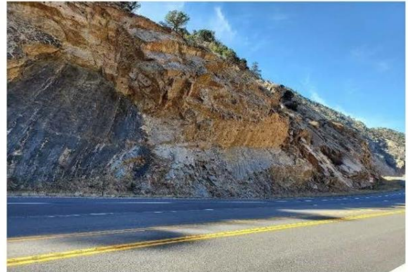
Westbound View, looking south-southeast at rock bolts, tilted rock
