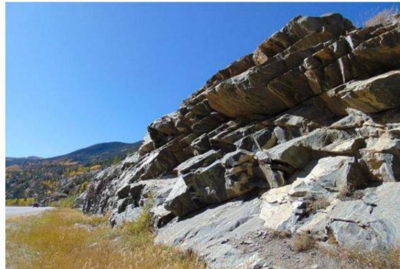
Joint planar surface dip toward roadway
