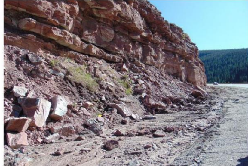
Boulders at base of slope and in ditch
