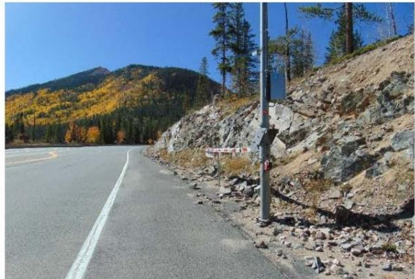
Soil cover and angular debris at shoulder, looking west
