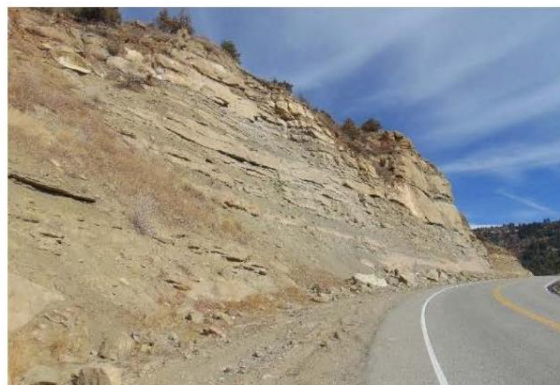
View to ENE, shotcrete lower slope, boulders up to 5 ft diam. In ditch
