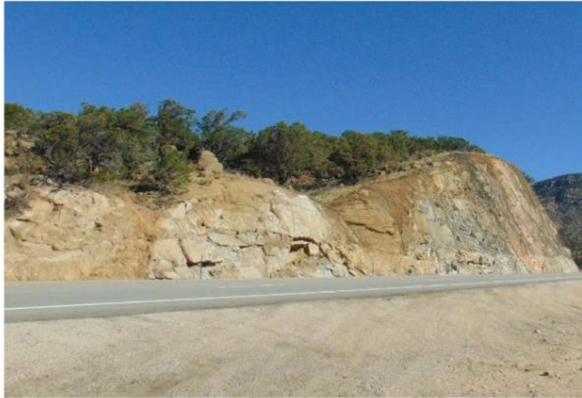
View to northeast, rock wedge missing
