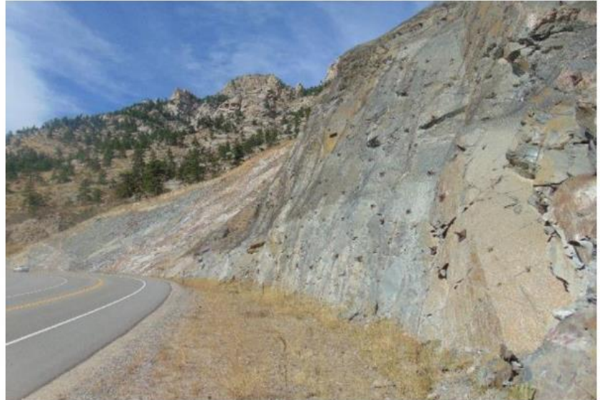
View to northwest, bolts, draped mesh, rocks caught behind mesh
