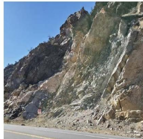
Looking south at loose rock on slope, boulder in ditch
